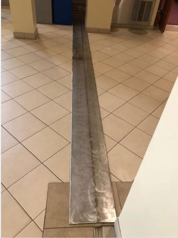
Stainless steel expansion joint cover installed in the gallery to protect the ceramic tiles
