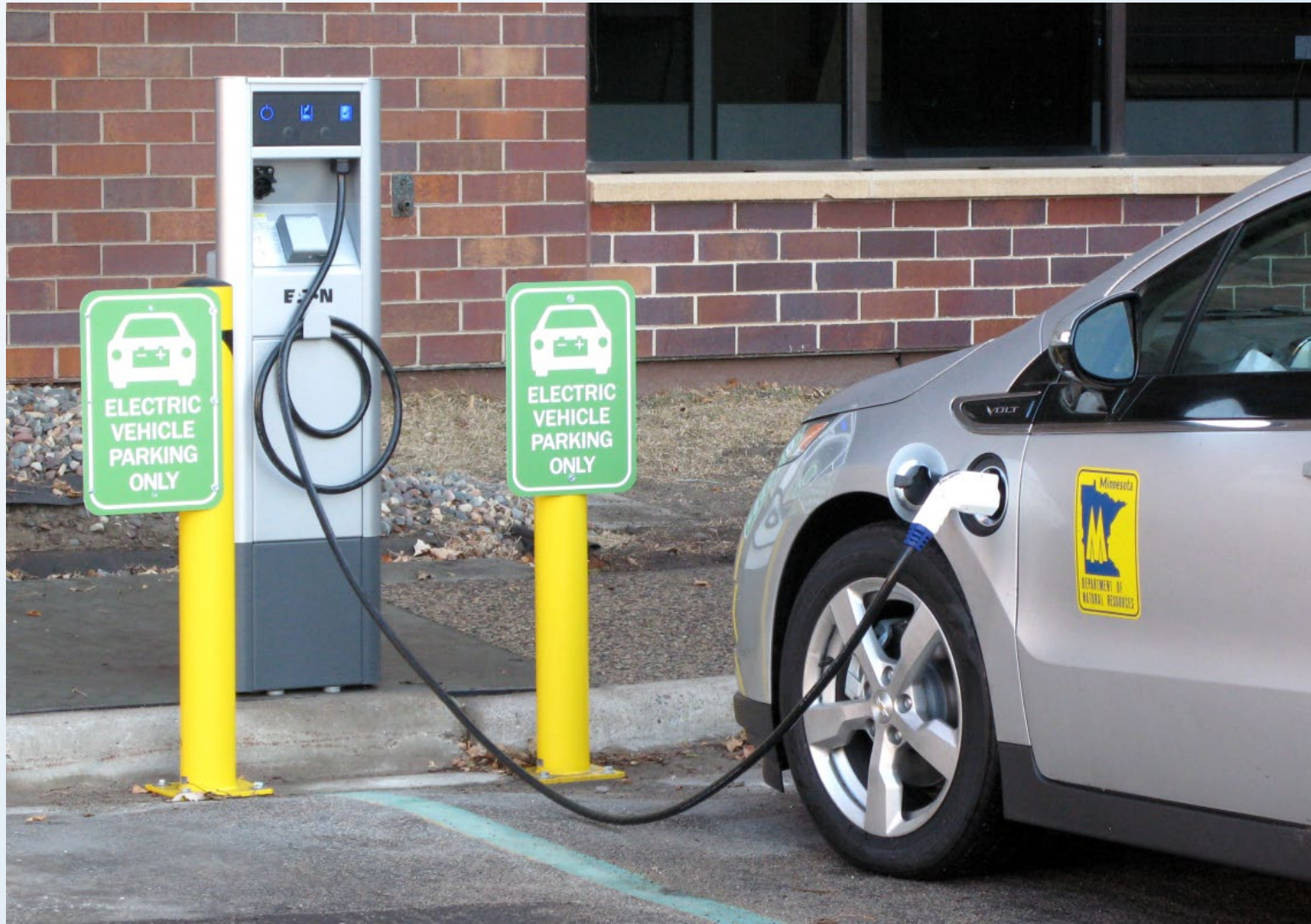
Electric vehicle charging station
