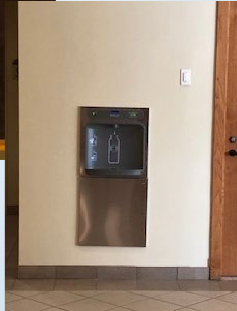
Charging and hydration stations
