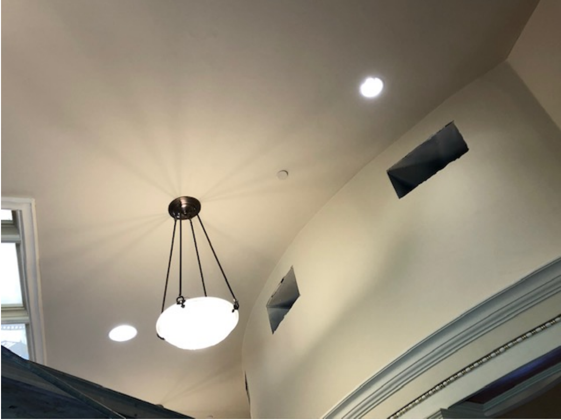
After: New plaster and paint have restored this area; the vent grilles are not yet reattached
