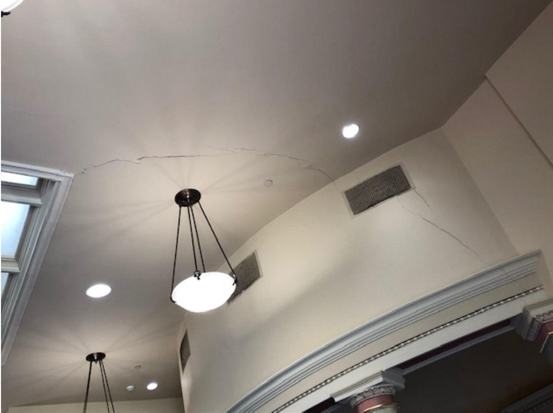
Before: Visible crack runs across the ceiling from the skylight to below the vent grille on the right
