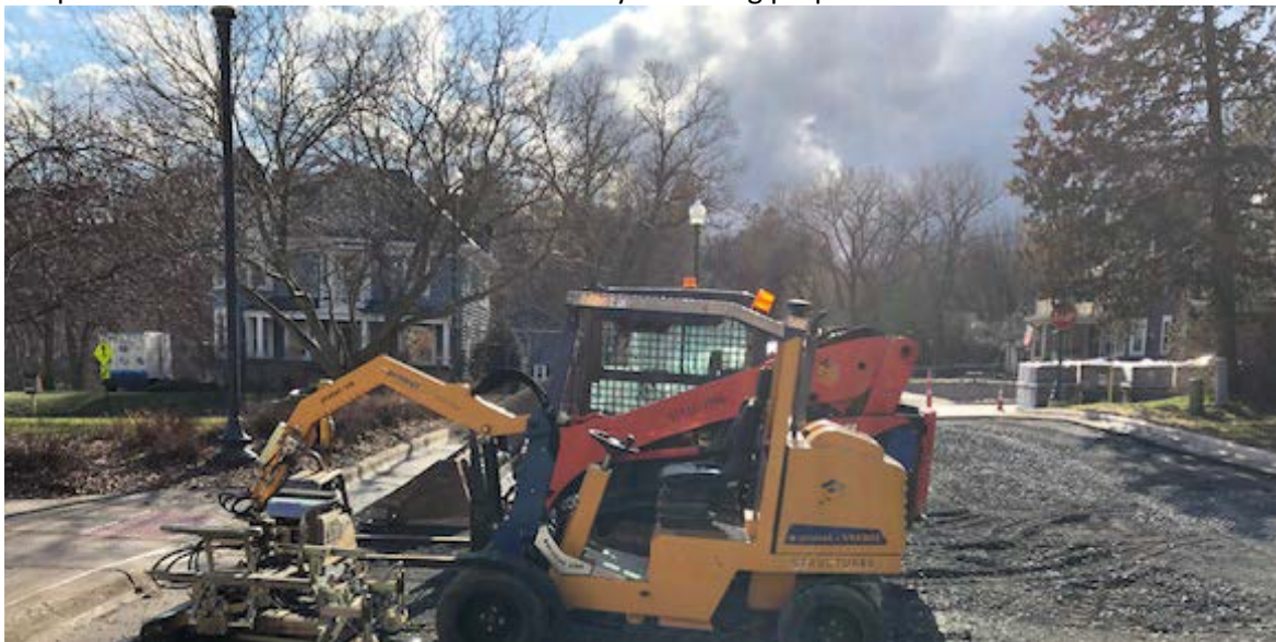
Old pavers have been removed and the base layer is being prepared
