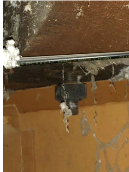
Photograph 5 Loose Tension Rod Nut
