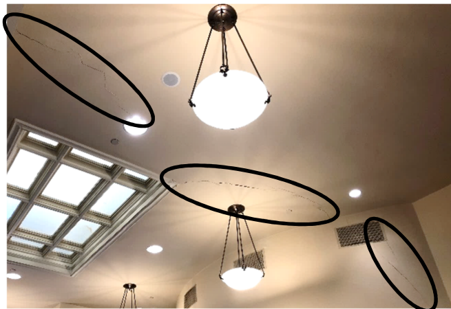
Photograph 1 Ceiling Cracks (highlighted)
